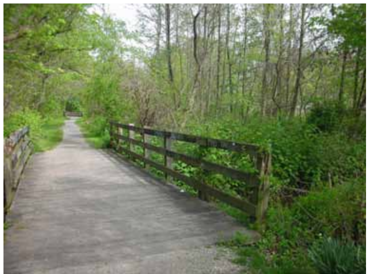
Possible sewage contamination
